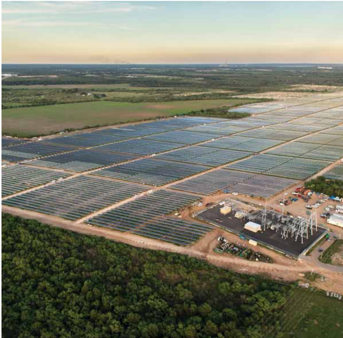
Investment in renewable energy sources, such as the Blue Wing Solar Project, are vital and will create a more resilient and sustainable San Antonio.
